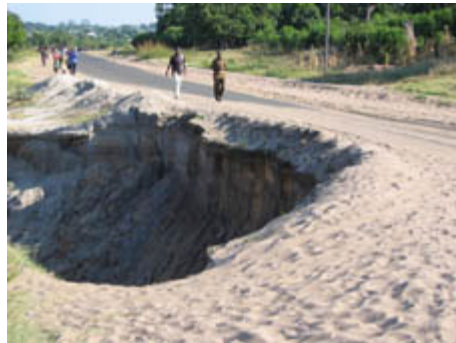
Washout in Main Road in Mongu
